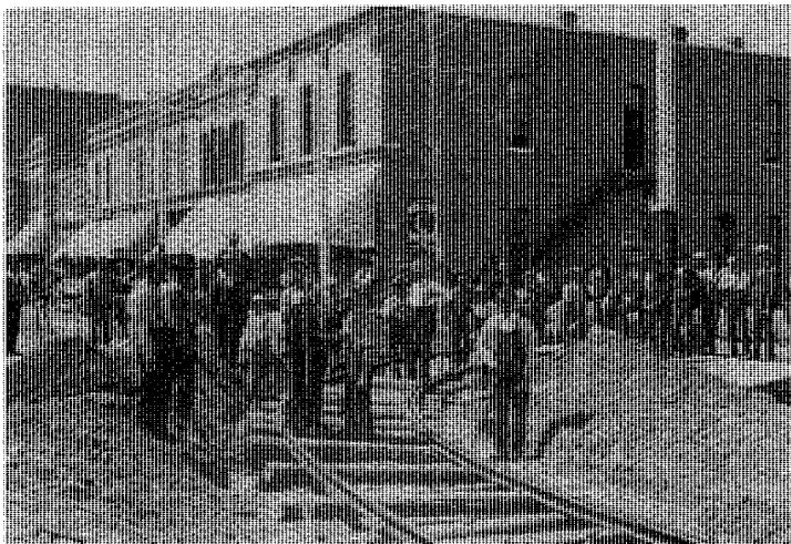
Waupaca Electric Railway tracks being laid through downtown Waupaca. Began running trolley cars on July 4, 1899.
